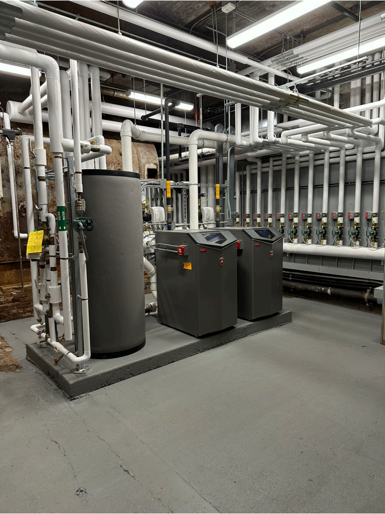
Updated new high efficiency boilers
